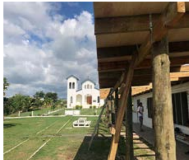
Church of the Holy Trinity during the construction of the new shed. FIJI
